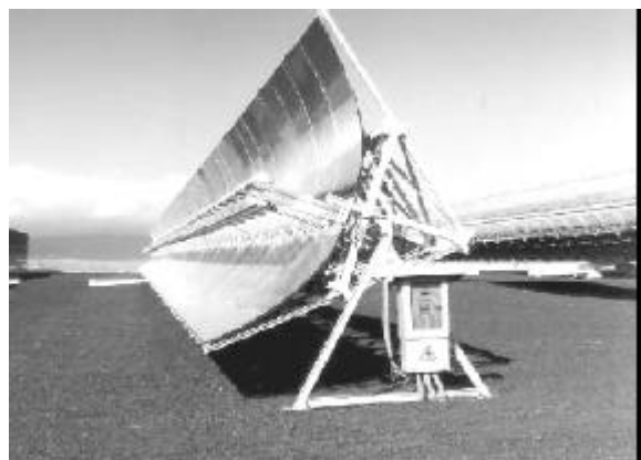
Figure 2: View of an array, with the tracking control box
